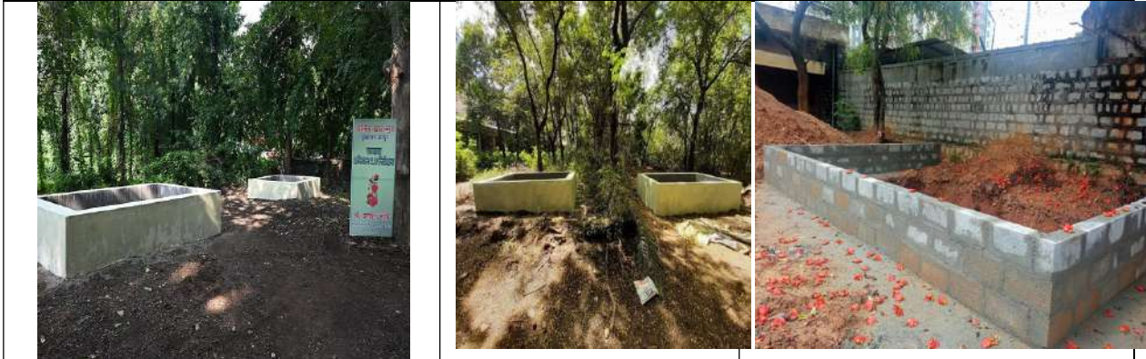
Compost Pit at IBM HQ, MMPL Hingana, IBM Bengaluru
