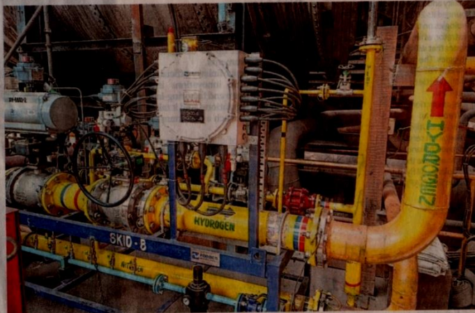
ADDED EFFECT. Piping hydrogen into a blast furnace requires careful handling to avoid leaks and embrittlement
